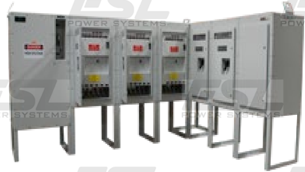
Concert Power Distribution Boards
